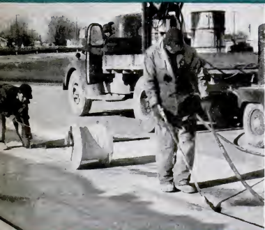
ELECTRONIC TRACK that automatically steers cars is simply cable, laid in \frac{1}{4} -inch saw-cut in concrete and then covered with asphalt. It emits weak radio signals along its length.
